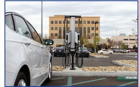
New charging station at 2100 Chester Ave.
