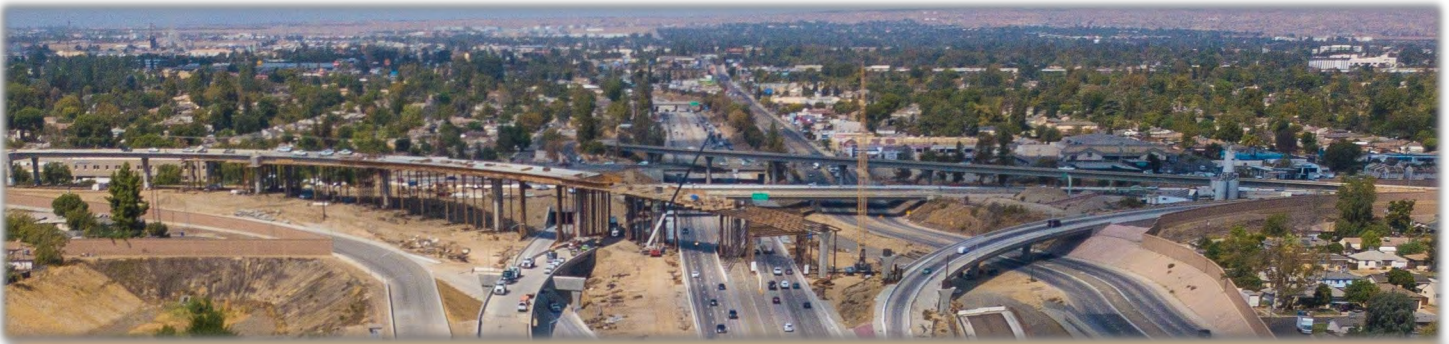
BAKERSFIELD FREEWAY CONNECTOR | LOOKING NORTH AT THE STATE ROUTE 58 AND 99 INTERCHANGE WHERE CONSTRUCTION EXTENDS THE 58 FREEWAY WEST AND BUILDS NEW RAMP CONNECTORS AND IMPROVES EXSTING RAMPS
