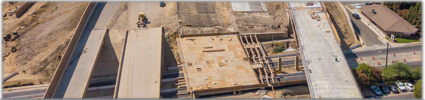
CENTENNIAL MAINLINE | LOOKING WEST AT THE NEW REAL ROAD UNDER CROSSINGS: FROM LEFT TO RIGHT THESE BRIDGES ARE (1) EASTBOUND 58 TO MING AVENUE OFF-RAMP, (2) EASTBOUND 58 TO SOUTHBOUND 99 CONNECTOR RAMP, (3) 58 EAST AND WEST MAINLINE FREEWAY, AND (4) NORTHBOUND 99 TO WESTBOUND 58 CONNECTOR RAMP. SEPTEMBER 2022
