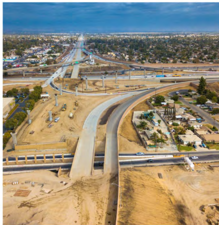
Centennial Mainline Real Road Bridges to various connector ramps. Looking east towards SR 99 & SR 58 September 2021
