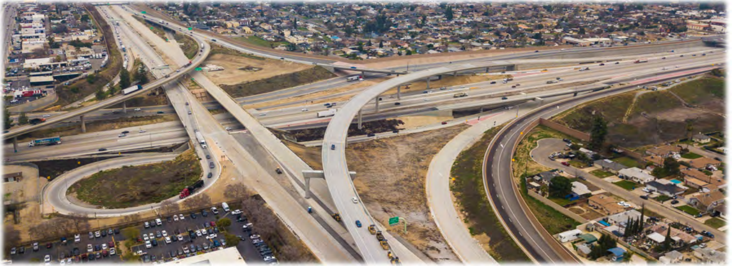
BAKERSFIELD FREEWAY CONNECTOR | LOOKING AT THE STATE ROUTE 58 AND 99 INTERCHANGE WHERE CONSTRUCTION EXTENDS THE 58 FREEWAY WEST AND BUILDS NEW RAMP CONNECTORS AND IMPROVES EXSTING RAMPS
