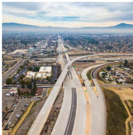
Centennial Mainline Real Road Bridges to various connector ramps. Looking east towards SR 99 & SR 58 January 2024
