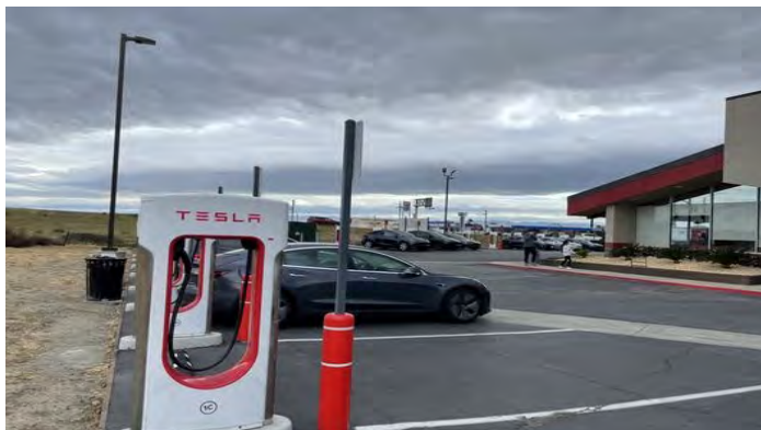
Electric charging station in Lost Hills
