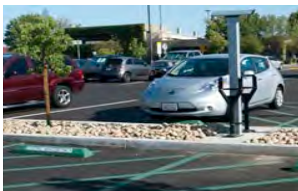
Electric charging station in Bakersfield
