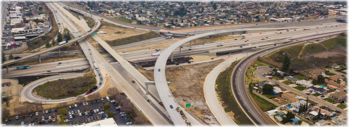
BAKERSFIELD FREEWAY CONNECTOR | LOOKING AT THE STATE ROUTE 58 AND 99 INTERCHANGE WHERE CONSTRUCTION EXTENDS THE 58 FREEWAY WEST AND BUILDS NEW RAMP CONNECTORS AND IMPROVES EXISTING RAMPS
