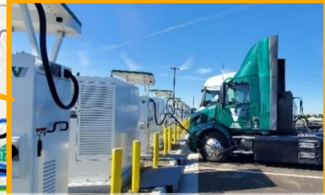
40 Truck Charging Units at WattEV Solar Battery Electric Off-Grid Truck Stop
